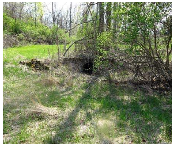
Photograph 2. Outlet structure for Willowbrook Basin (BMP A7)
