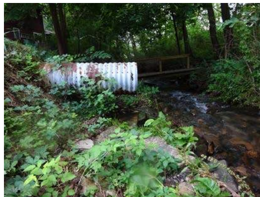
Photograph 3. Eroded streambank upstream end of reach
